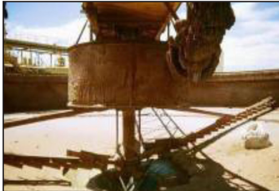
Thickener discharge cone
